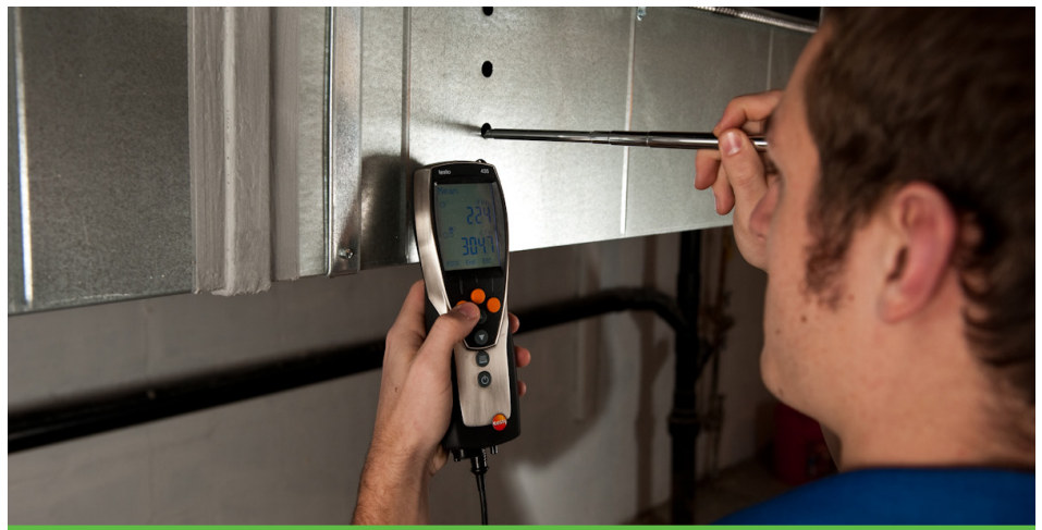
HVAC SAVE Certified Contractor Measuring Airflow Photo courtesy of the Midwest Energy Efficiency Alliance (MEEA)
