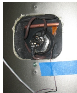
Figure 20. Surface-mounted TC at the lower tank surface
