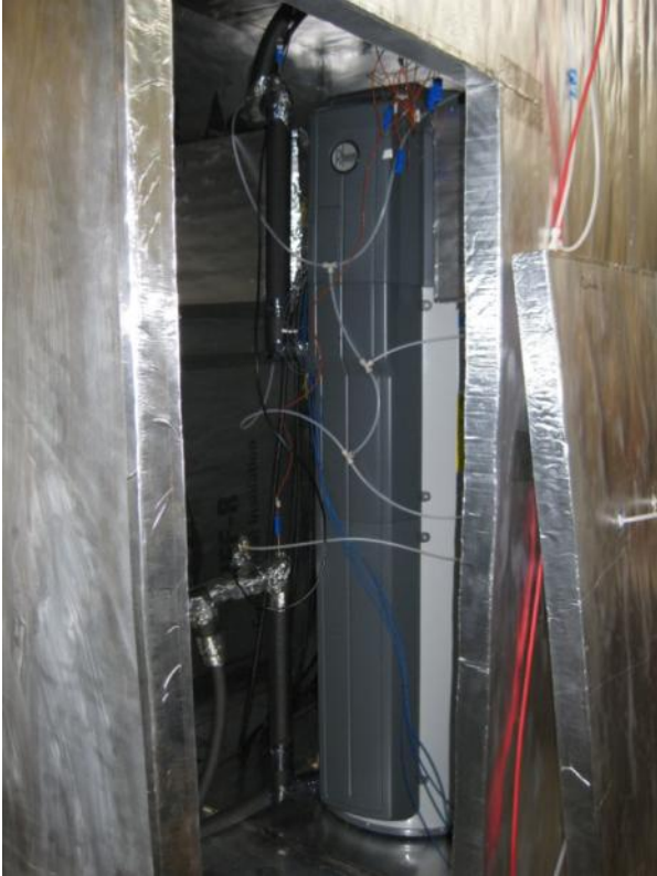
Figure 2. EcoSense Installed in Test Chamber
